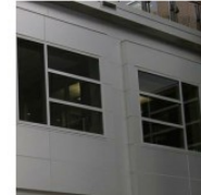
3. PREFABRICATED EXTERIOR CLADDING METAL PANEL SYSTEM - SINGLE TONE CUSTOM COLOR PAINT ON METAL PANELS
